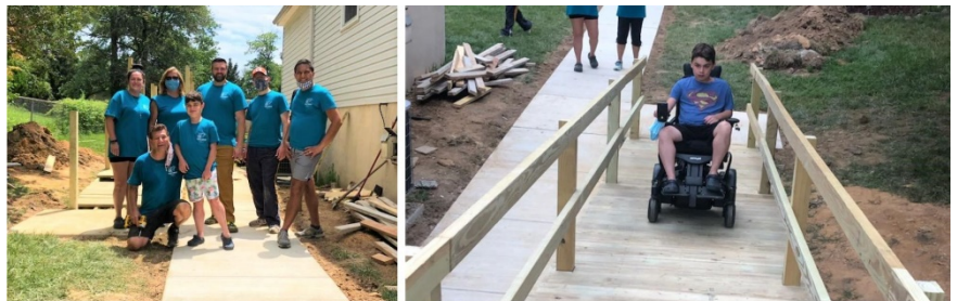
COVID-19 didn't stop our passionate associates from getting out and helping the community. Rockville, MD associates volunteered to build an access ramp for a family in need, funded by Choice's Associate Grant Program.
