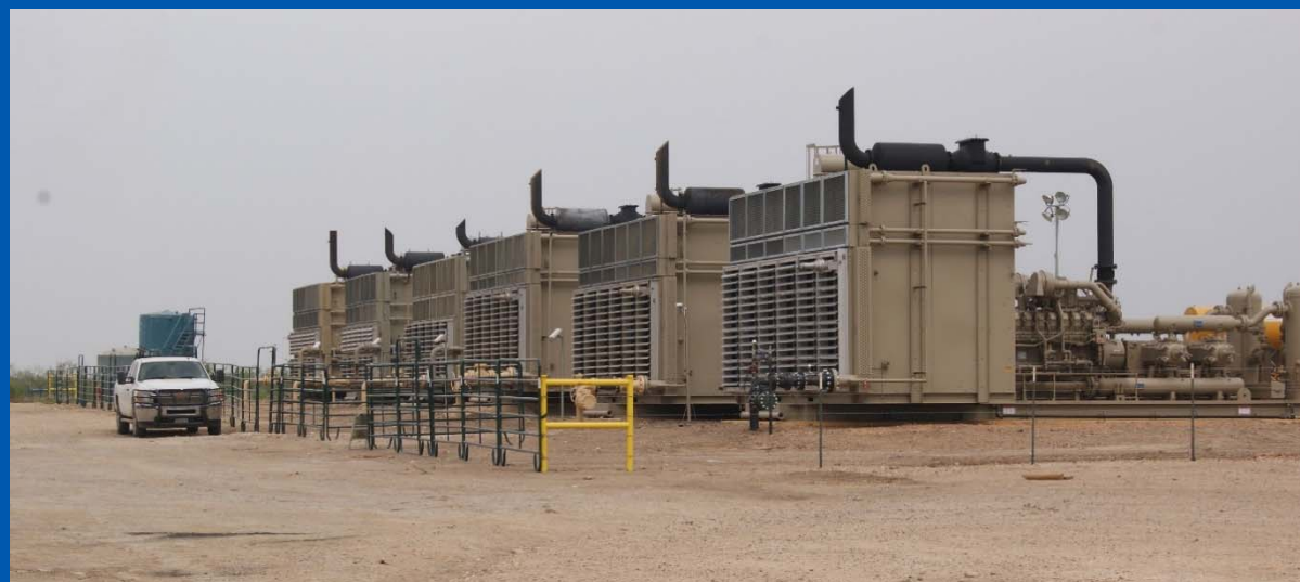
8,160 Hp Booster Station Webb County, TX
