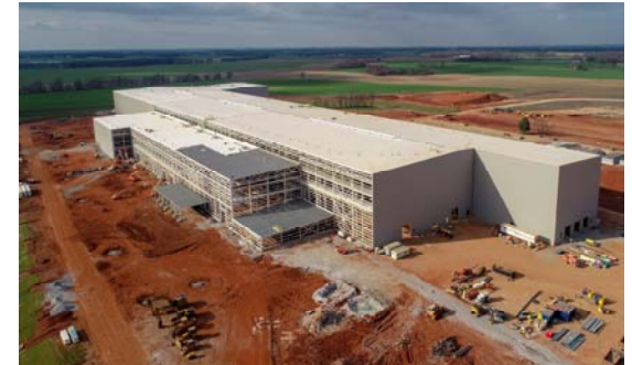
Greenfield finishing line in Guthrie, Kentucky
