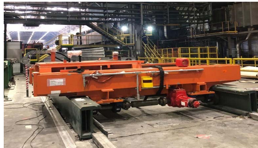
Coil handling system equipment on site in Pinda
