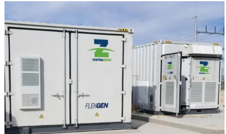
Upton 2 Energy Storage Facility
