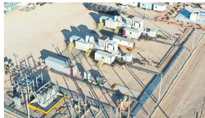
Pictured: APR gas turbine deployment in La Rosita, Mexicali
