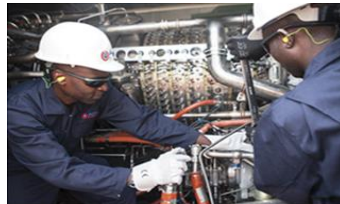
Pictured: APR personnel maintaining an aeroderivative turbine
